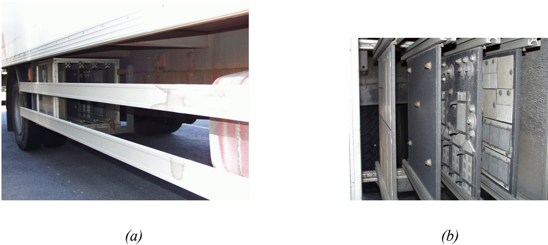
Figure 2: a) The field test by placing a) plates and bolts under the chassis of a truck. b) The corrosion surfaces of plates parallel with the driving direction.
